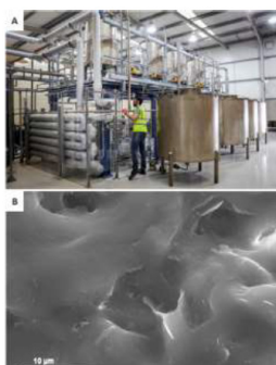
Figure 1. (A) Promethean's multi-ton scale nanoparticle manufacturing plant (capacity more than 1000 tons per year),(B) SEM image of a bioglass-based material.
