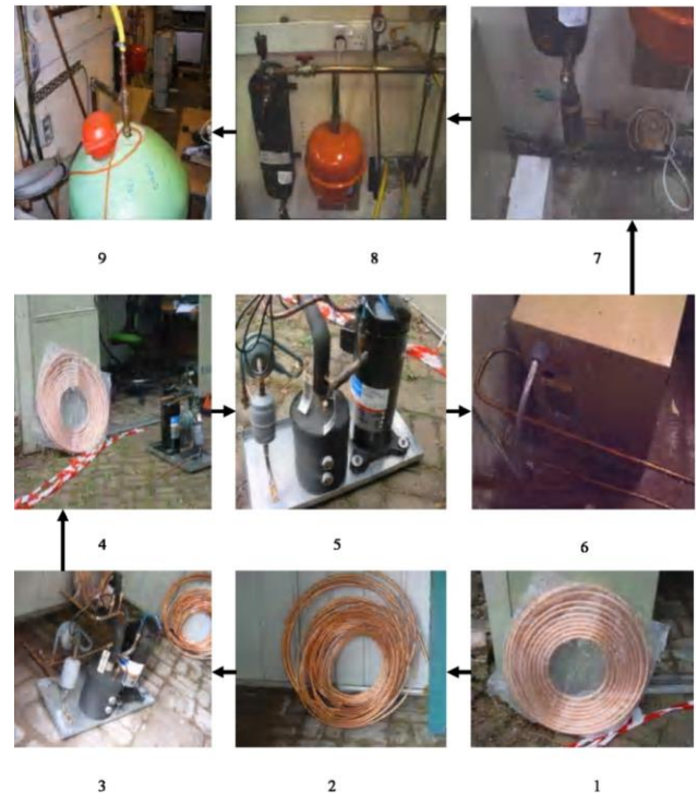
Figure 4) Showing preparation of coils in 1 and 2, installation of a heat pump in 3 to 6, and connection of water supply system (water pump, flow meter, expansion valve, and the boiler in 7 to 9
